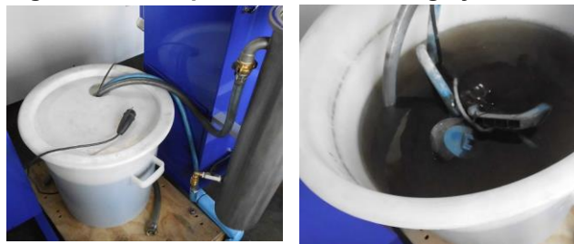
Figure 11: example of second cooling system
