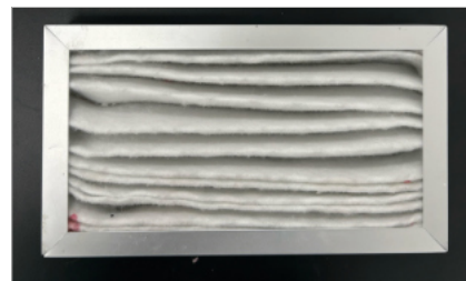
Filter to be replaced
